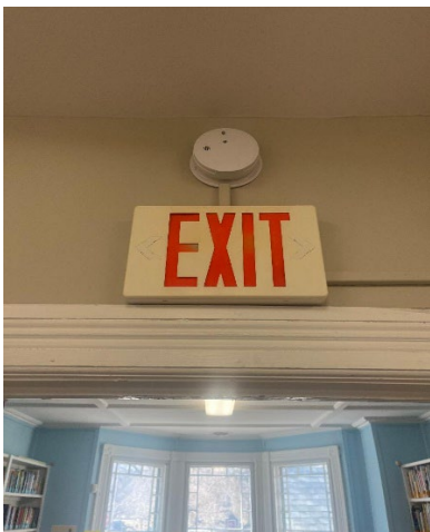
Smoke Alarms X3
