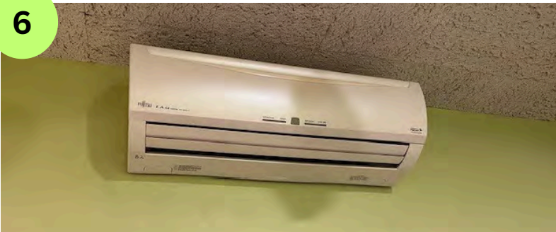
Mini split in office. Doesn't drip much, but no cooling either. Room not used much anyway, except by Library Director.
