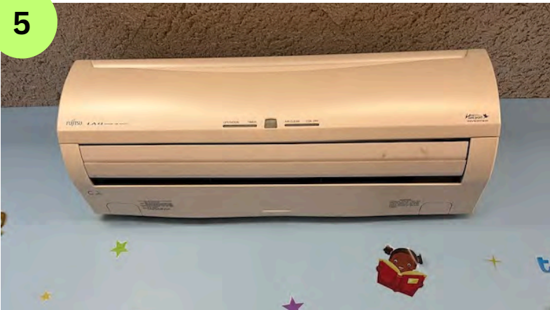
Mini split in kids' room. Not one of the worst drippers but not very effective at cooling.
