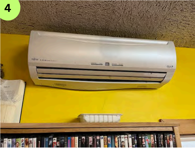
Mini split across from circ desks. Tray placed under to catch drips & protect shelves under.
