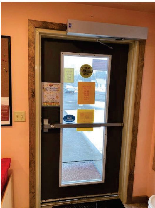
Photo 3: Inside of door showing the now defunct opening mechanism.
