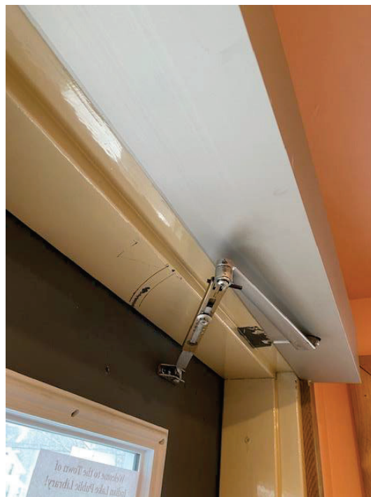
Photo 4: The bracket that kept being overextended, broken, and repaired by turns.
