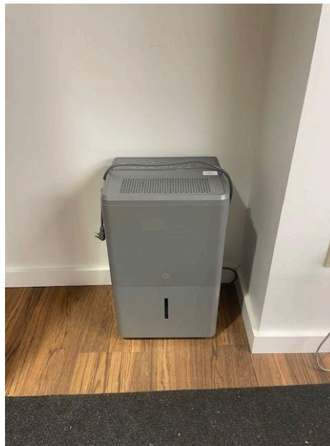
Temporary portable humidifier, in Gill Room
