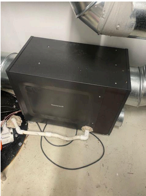
Broken Humidifier, in furnace room
