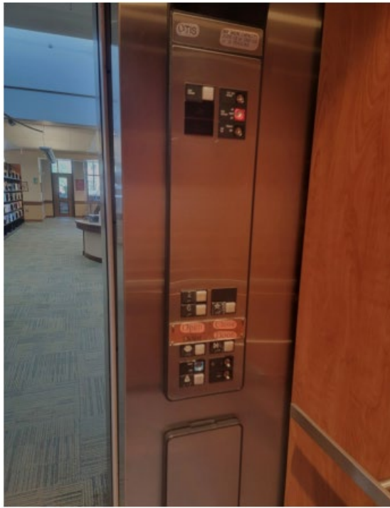
Interior Elevator Controls
