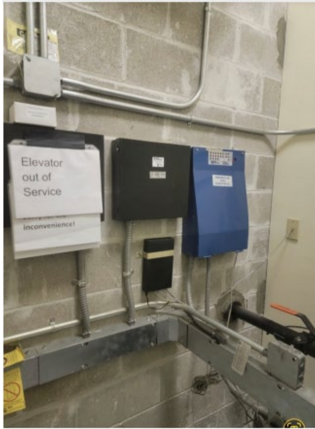
Elevator Control Room
