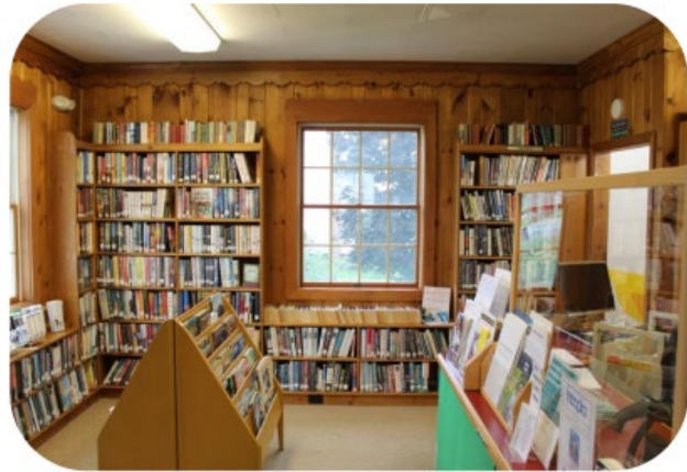
Easton Library: Interior, Window where the new doorway to the children's room addition will be
