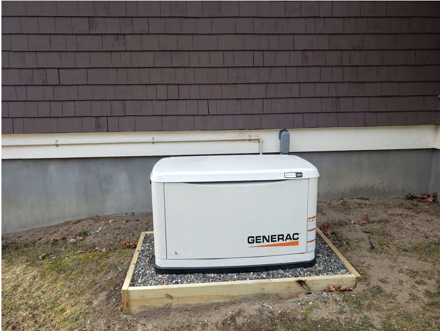
Bolton Free Library Outside Generator February 2024
